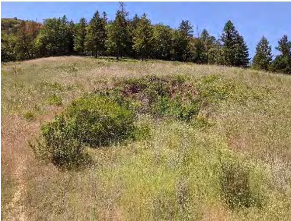
P05 – Erosion/hill slump looking west
