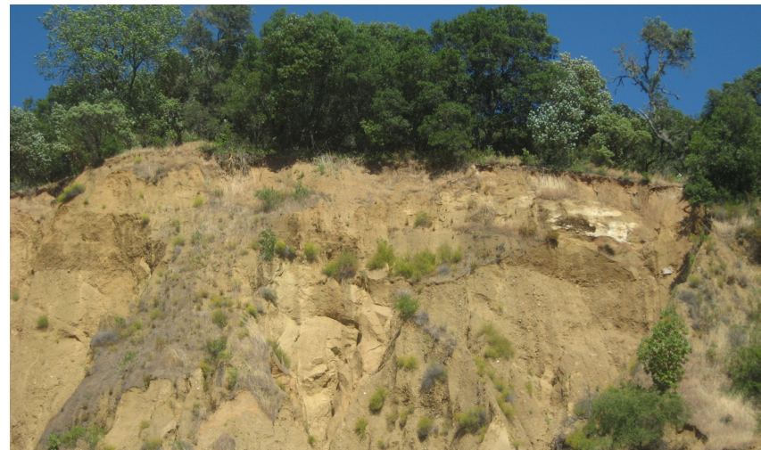
Areas at high risk of erosion along Redemeyer Road.
